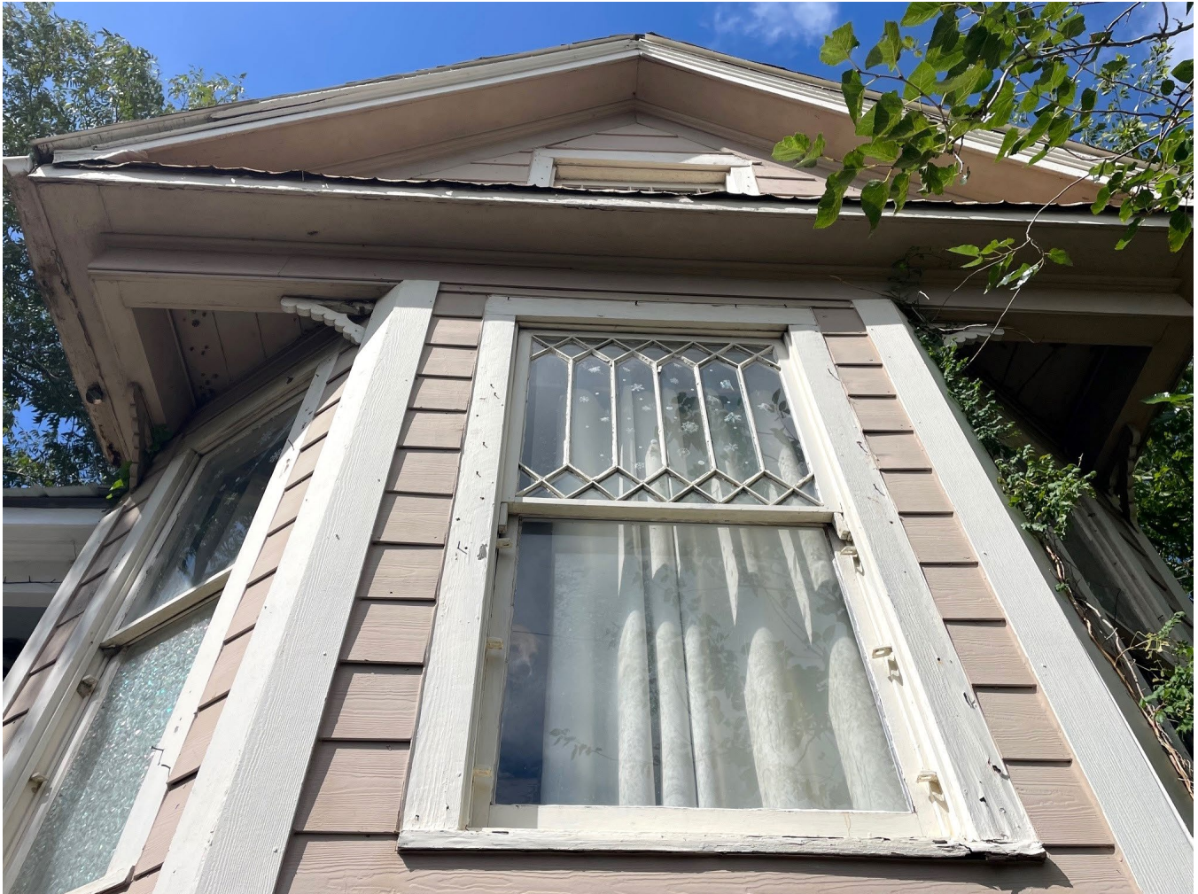
Photo 7: Close-up detail view of original Queen Anne window on the primary east elevation. Photo by HOP staff member, Cara Quigley, October 6, 2023.
